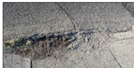
Figure 19 - Missing Truncated Domes and Curb Ramp in Poor Condition
